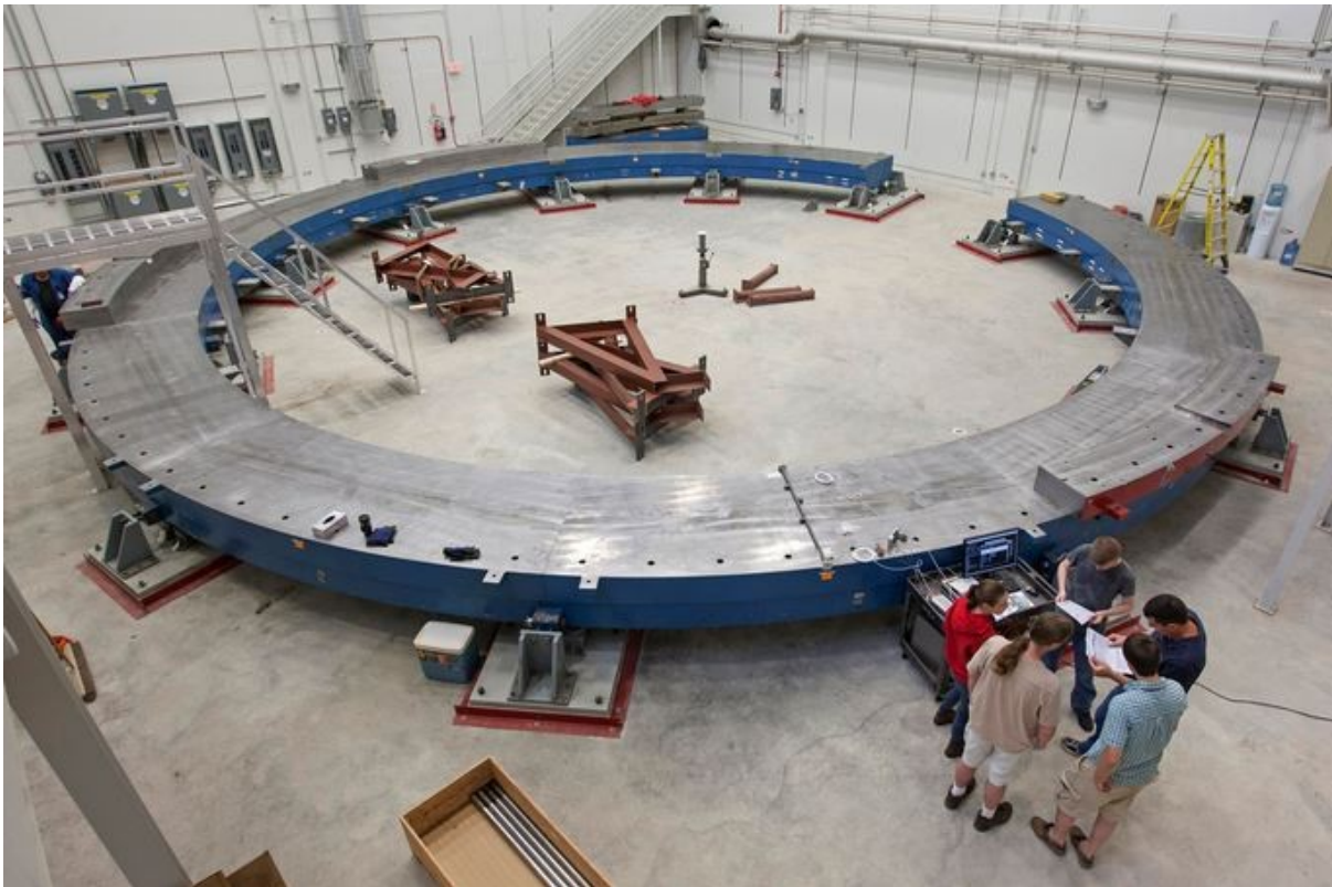
Figure 3.8: Yoke placement in progress in the MC-1 building at Fermilab. (Image courtesy of Scott Walstrom, NIU).
